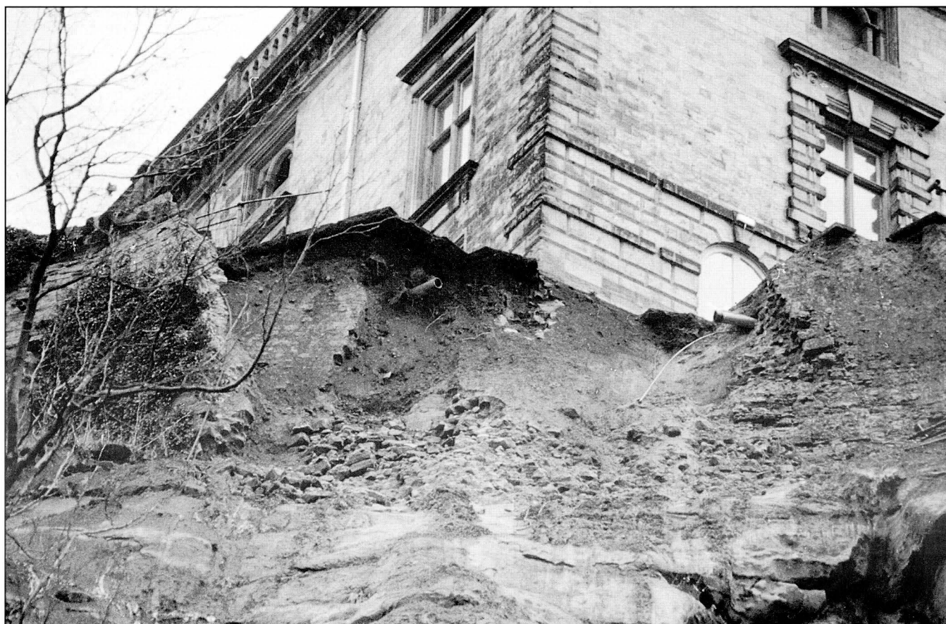
Closer view of the slide scar, with the masonry of the Norman wall visible beneath the overhanging terrace paving; undisturbed sandstone is exposed at the foot of the picture.
